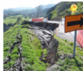
Head-scarp of a slump (California)
