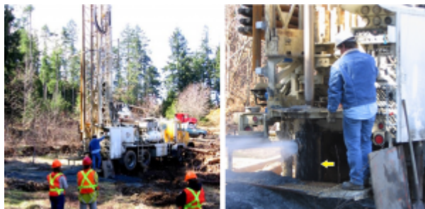
Figure 14.10 A water-well drilling rig in operation in the Cassidy area, near Nanaimo, B.C. In the photo on the right the well is being test-pumped with air pressure. The casing (yellow arrow) is about 40 cm in diameter. [SE]
