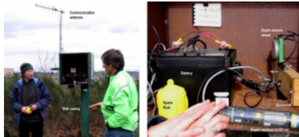
Figure 14.13 B.C. observation well 232 near Cassidy Airport, Vancouver Island. The installation also has a solar panel, which is not visible in this view. [SE]
