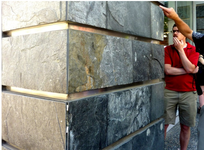
Figure 20.17 Slate used as a facing material on a concrete building column in Vancouver [SE]
